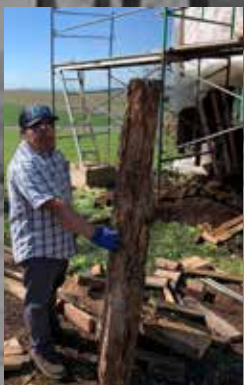
Ioka employee Efrain Hernandez holding a rotten sill board.
