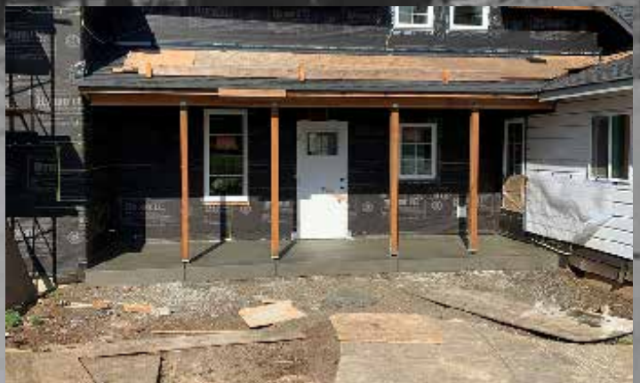
The same porch after adding footings and a foundation. The porch was sagging and also needed to be rebuilt.
